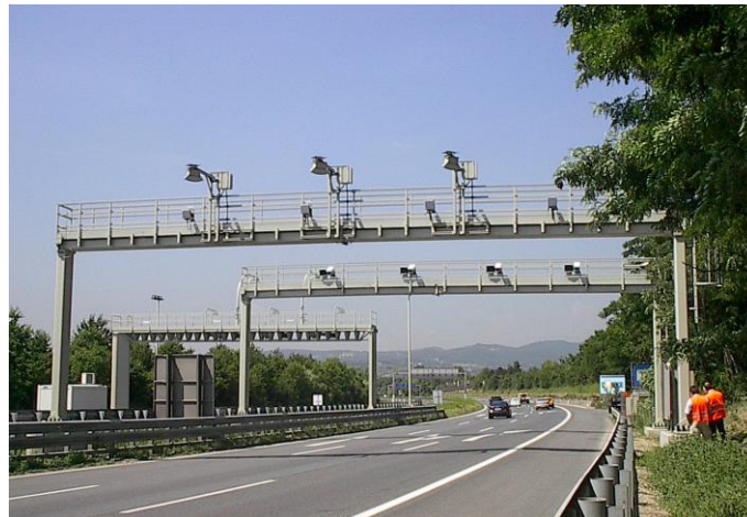
Figure 4: Enforcement station for Austrian HGV toll scheme
